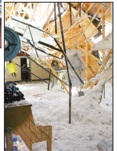
Photos courtesy of The Huntsville Times DAMAGE — Insulation covers the gym floor of Wall Highway Baptist’s CLC following the roof collapse.
