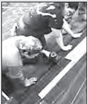
Photo courtesy of Metro Changers Metro Changers volunteers repair the roof of a home.
