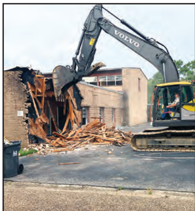
Photo courtesy of FBC Chickasaw Demolition begins on First Baptist Church, Chickasaw's, office and fellowship hall.
