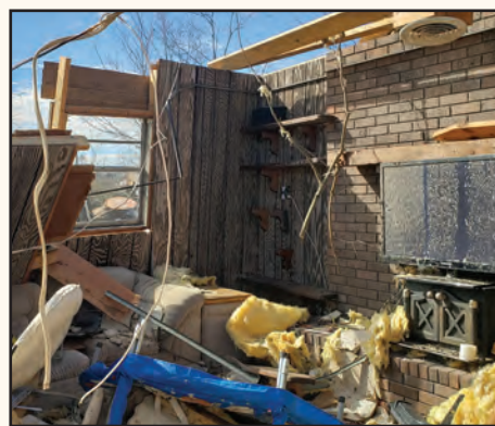
Photo by Cynthia Walker Watts A tornado tore away the roof and most of the walls of Jean Hadley’s home in Fultondale on Jan. 25.
