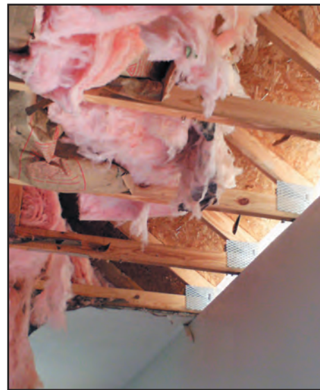
Photo courtesy of Pilgrim Rest Baptist Church The building of Pilgrim Rest Baptist Church, Centre, was destroyed April 27, 2011, when a tornado lifted it off its foundation.
