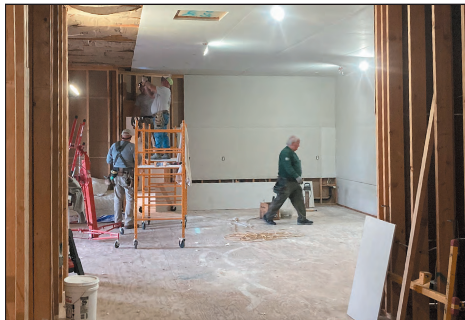
Photo by Beth Baldwin Volunteers from FBC Tallassee install drywall in a future Sunday School classroom at Liberty Baptist Church during a missions trip to Craig, Alaska.
